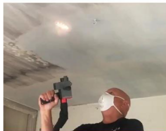
Fire Damage Restoration
